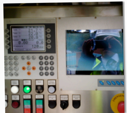
UV CONTROL PANEL
